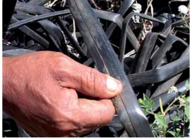
'Good stuff' but bad installation. The tank is too low and would require pumping water 8 hours a day with a rope pump
