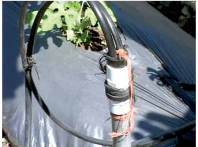
Supply chains are very weak. Good equipment is available, but mainly in the capital. Spare parts are often scarce
